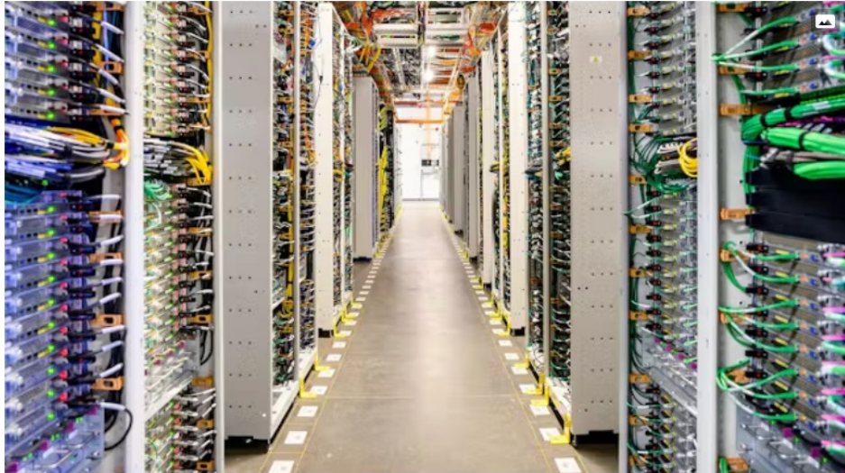
Project Rainier Server and Cable Installation
